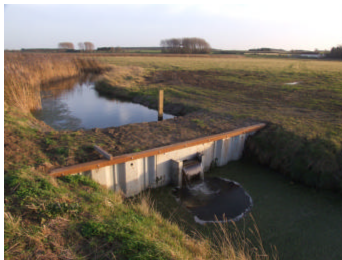
(Above) – the main outlet drop board sluice at Deepdale Marsh allows for ditch and field water levels to be set across the whole site.
