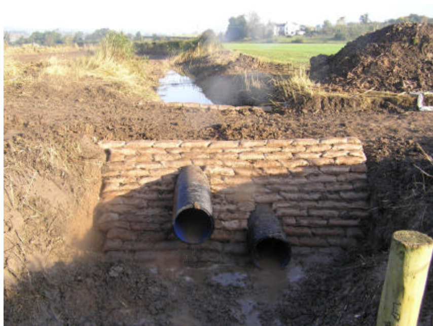
(Above) – main water outflow via a split level sluice as seen during construction at Poulton Court
