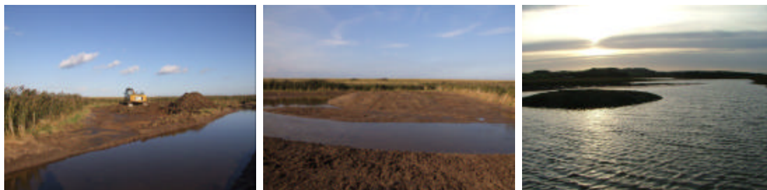
(Above) – creation of a new island and surrounding shallows prior to water level management at Deepdale Marsh, Norfolk
