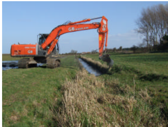
(Above) – restoring an old overgrown ditch at Deepdale Marsh, Norfolk prior to re-profiling and new water level management.
